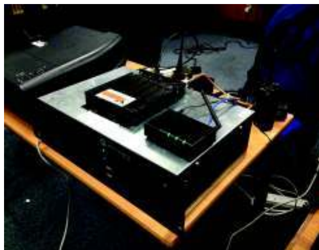
A DMR base-station and link to internet
