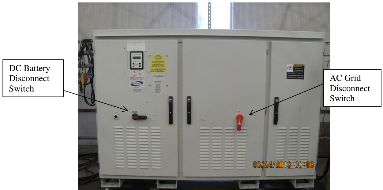
Figure 3-1: DC Battery and AC Disconnect Switch Shown in the On Position
