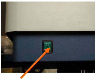
Evaporator power switch
