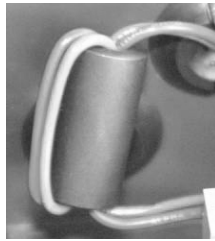
Figure 2-5: Ferrite core and battery supply wiring
