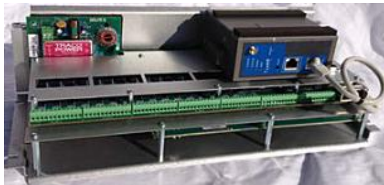
Figure 1 - 3. SKF Multilog On-line System IMx-B, Inside.
