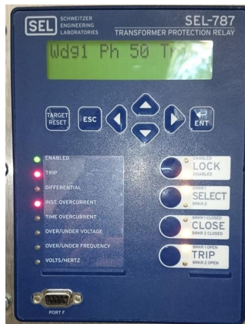
Figure 26 – Fault event SEL-787 Front Panel
