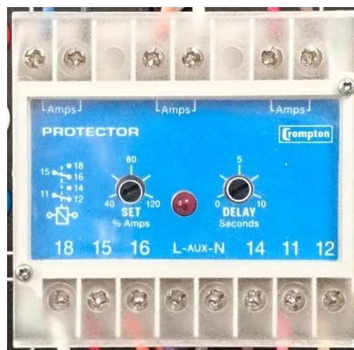
Figure 4 - Three-Phase Overcurrent Relay
