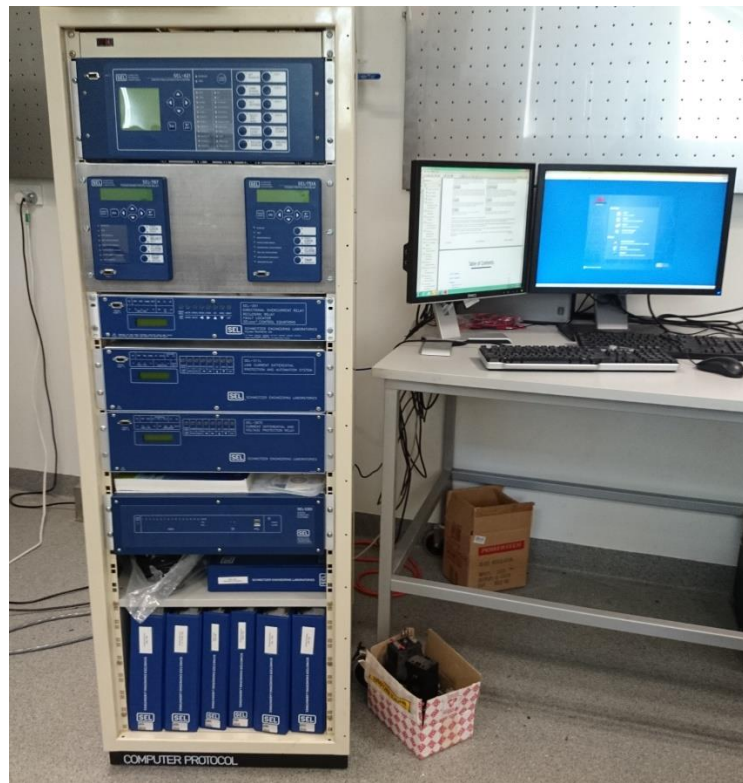
Figure 2 - SEL Protection and Monitoring Rack
