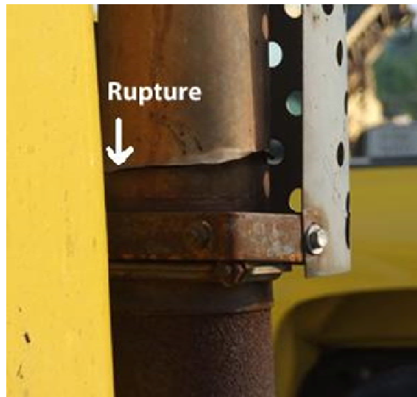
Figure 25. Ruptured Tailpipe of Truck 5715 from the B20FA run on July 8, 2009
