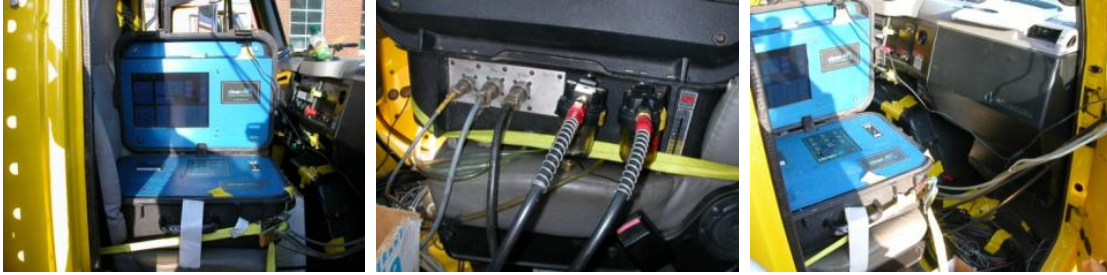
Figure 20. Installation of the Portable Emissions Measurement System (PEMS) Main Unit in a Truck 215-5715:
