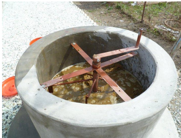
Photo A-1: Inlet Tank for Mixing Water and Manure
