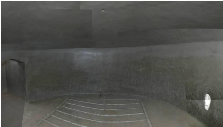
Photo 14.2: Panoramic View of Plant Interior with Solar Water Heater Manifold on Floor.
