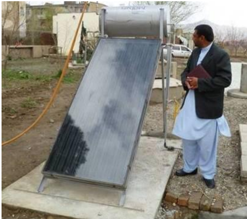
Photo 14.1: Solar Water Heater for Biogas Plant.
