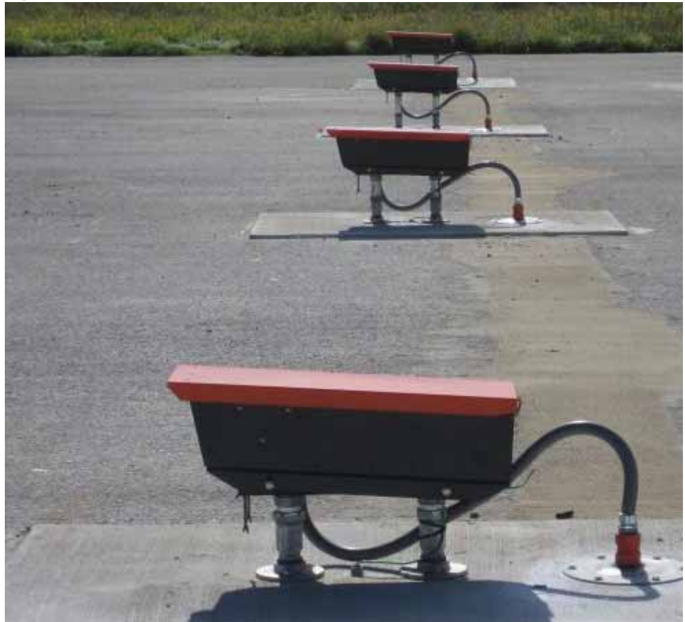
Figure 9: Example PAPI Installation
