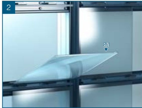
2.1. The glazing panels can now be placed into the openings. Ensure care is taken to position glass correctly & squarely within each opening & onto the glass setting blocks.
