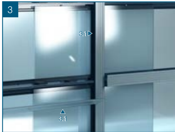
3.1. Once glass is in place, the vertical pressure plates can be positioned over the PVC spacer. Ensure the appropriate gaskets have been inserted.
