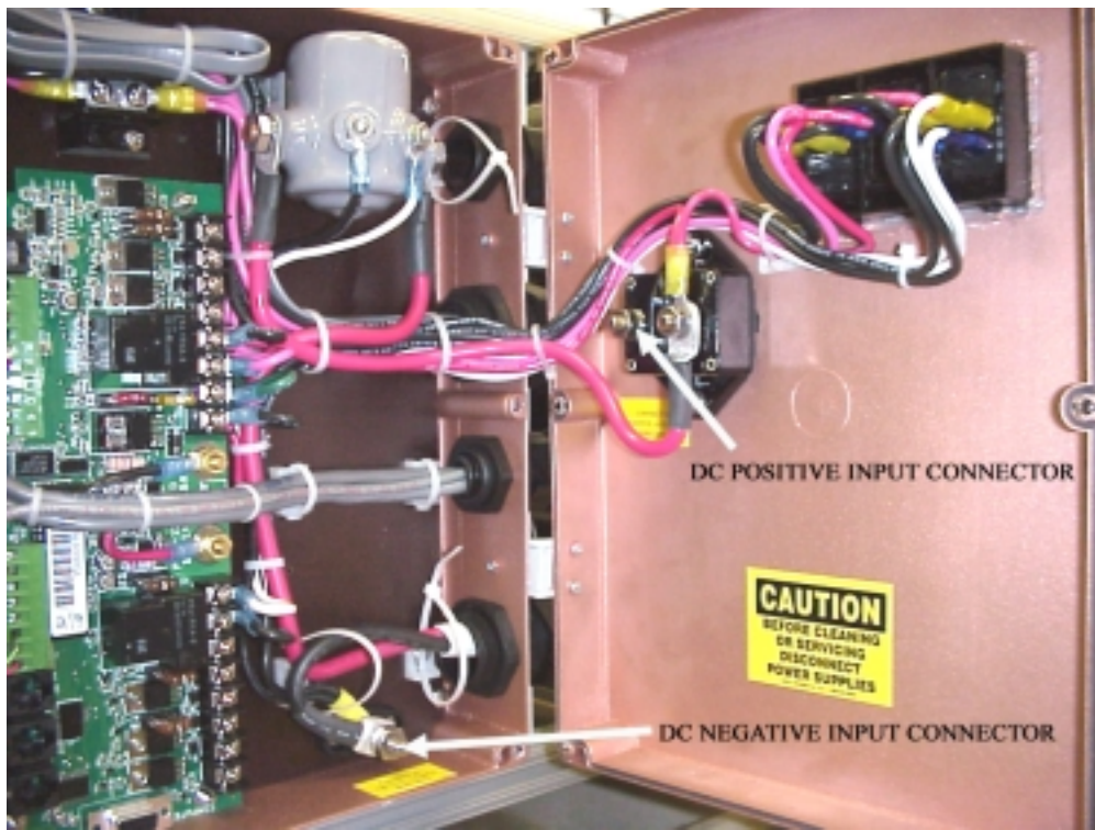
DC Powered Feed Pump Connections
