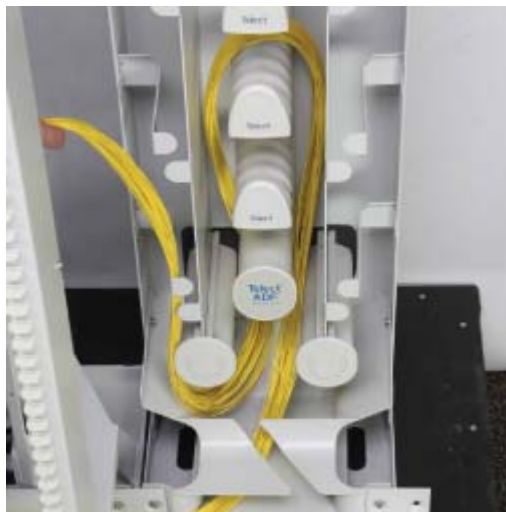
Figure 25 - Storing Excess Cable
