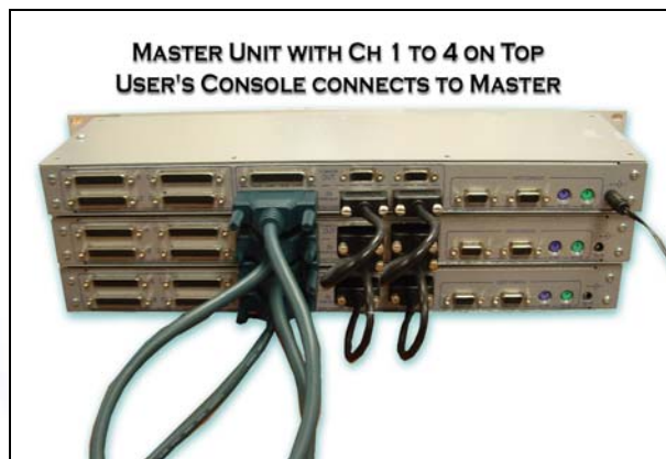
FIGURE 3 Stacking of MC4-H2 Units
