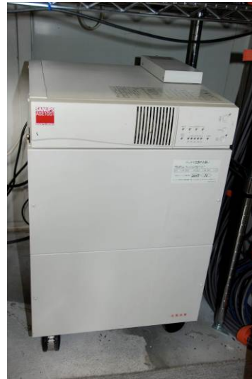
Photo 2.7-3 Uninterruptible power supply unit (UPS).
