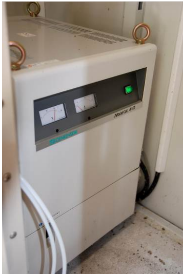
Photo 2.7-2 Noise cut transformer for power supply.
