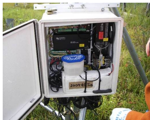
Photo 1.2-13 A measuring box with desiccant (closet dehumidifier) inside.
