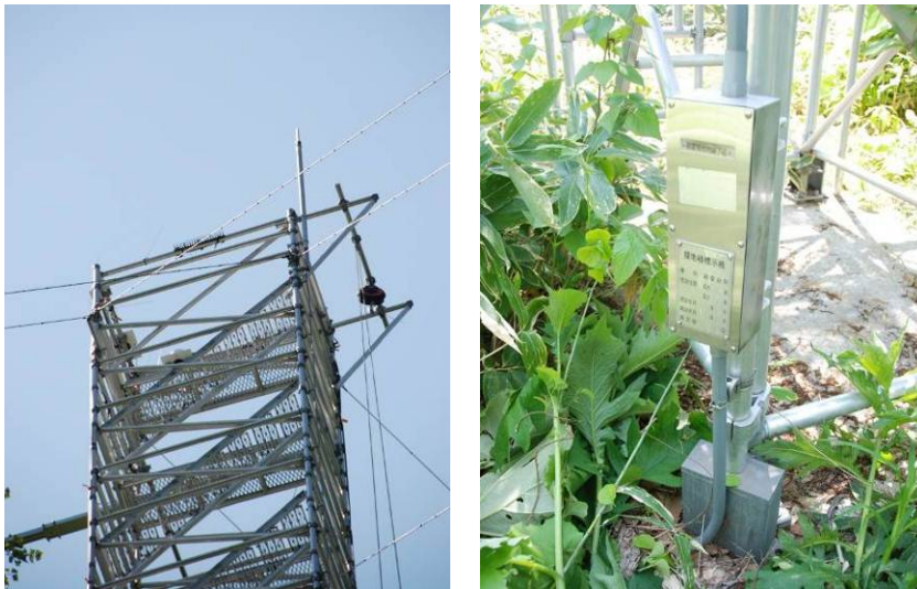
Photo 1.2-9 A lightning rod (left) and a ground (right) installed in an observation tower. (Sapporo forest meteorology research site)
