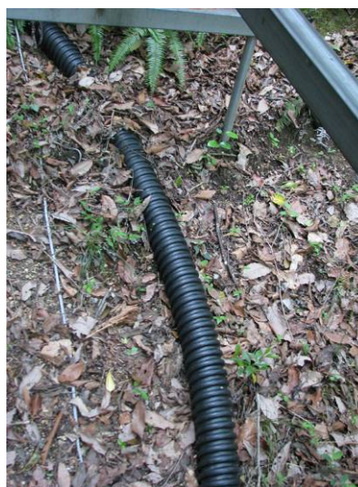
Photo 1.2-7 Unfixed wiring. The forest floor undulates, so it is more practical to use underground corrugated protective tubes for unfixed wiring. (Yamashiro forest hydrology research site)
