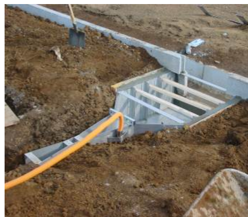
Photo 3.8-3 An example of installation of a Parshall flume for the measurement of the flow rate of an open channel flow. (Photograph: Courtesy of Senecom, Inc.)
