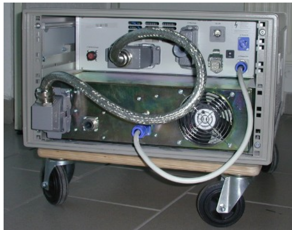
Connections: Data, Temperature, Heater Power, Interlocks, Warnings, HV PSU monitor and control, relay switched mains power out, mains power in.
