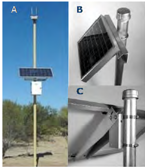
Figure D.4. Control box and solar panel mounted on pole.
