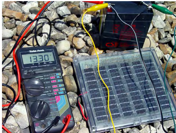
Figure 4.10: Solar panel, meter, and battery
