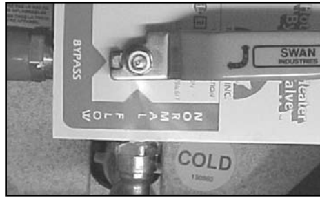
HOT WATER TANK BYPASS VALVE
