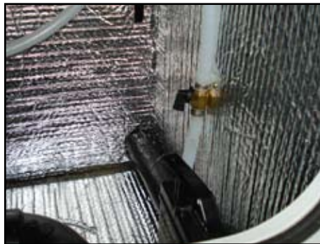
LOW POINT DRAIN VALVES
