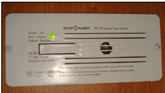
LP GAS MONITOR
