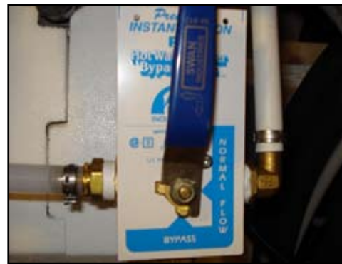
HOT WATER TANK BYPASS VALVE
