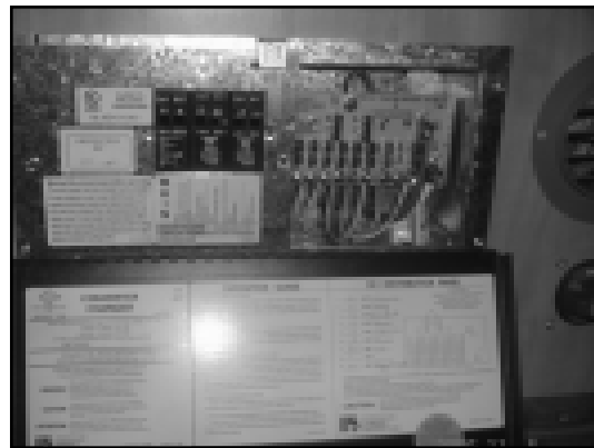
120 VOLT CIRCUIT BREAKERS AND 12V FUSES
