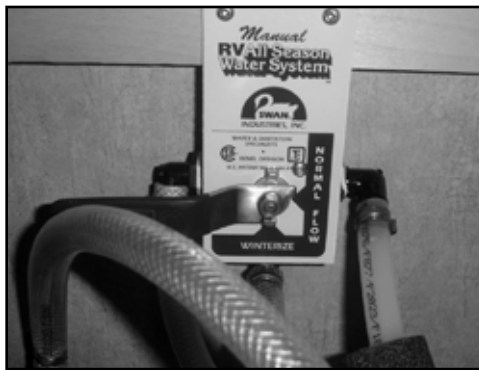
ANTI-FREEZE BYPASS VALVE
