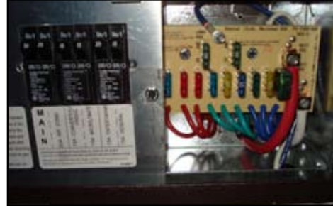
120V CIRCUIT BREAKERS AND 12V COACH FUSES
