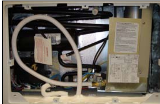
EXTERIOR FRIDGE ACCESS
