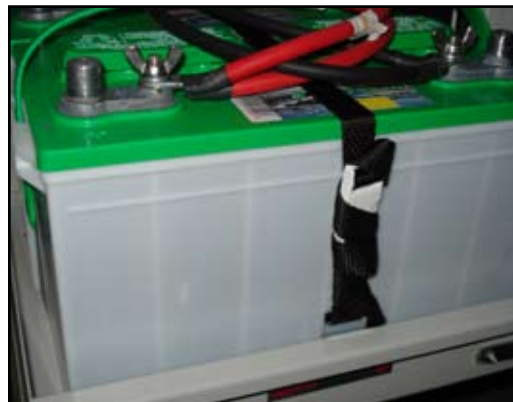
COACH BATTERIES USUALLY IN AN EXTERIOR COMPARTMENT; COULD ALSO BE UNDER ENTRY STEP.
