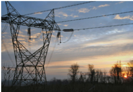
Electricity Transmission Cables
