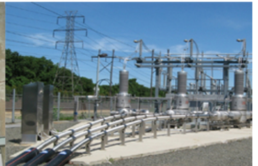
Power Distribution Grid
