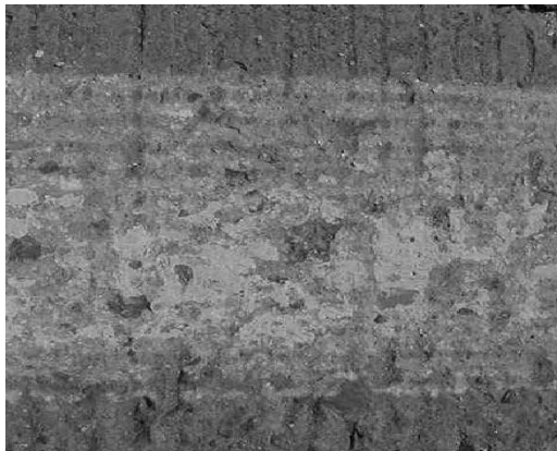
Figure 2 — Poor removal — Need to slow equipment down to remove more of the existing marking.
