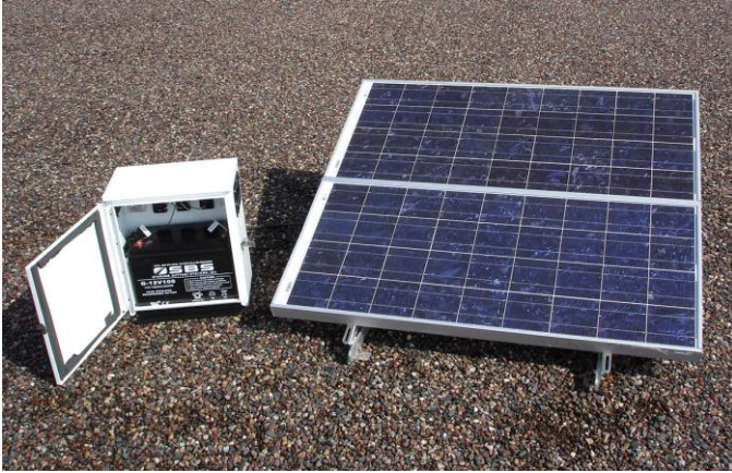
Figure 38: Solar Cell Power System
