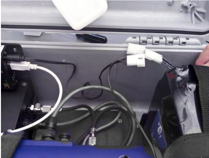
Figure 36: Internal DC Power Connections
