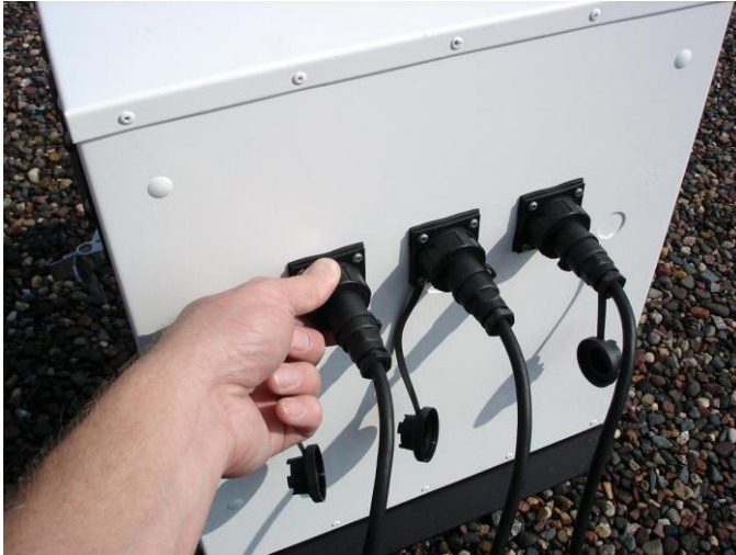
Figure 48: Connect Power from the Solar Cell Power System to the Environmental Enclosure
