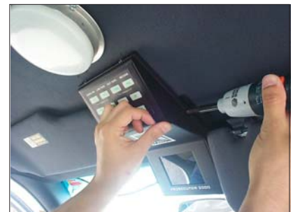
View of control head being mounted with wires already attached to connections
