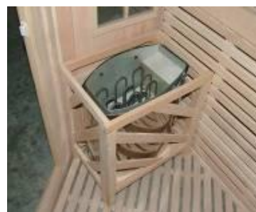
FIG-26 location of the stove
