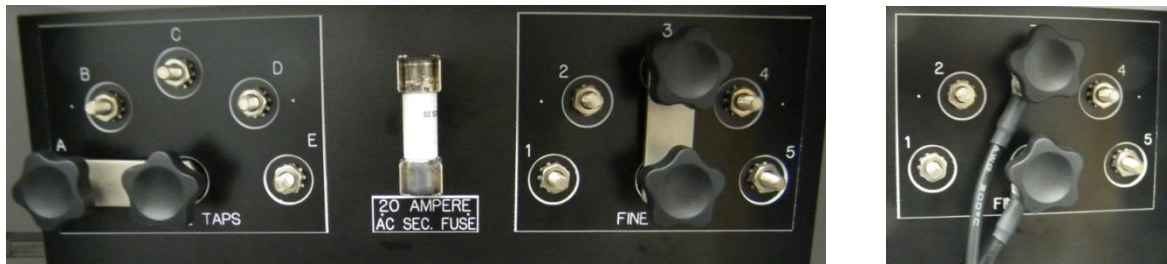
Figure 17 SRL1 Relay Contacts Installed In Series With Taps (Tap Bar Removed While In Use)
