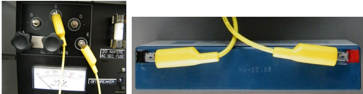
Figure 15 uGI1 Power Connections (AC voltage from rectifier taps or DC voltage connections)
