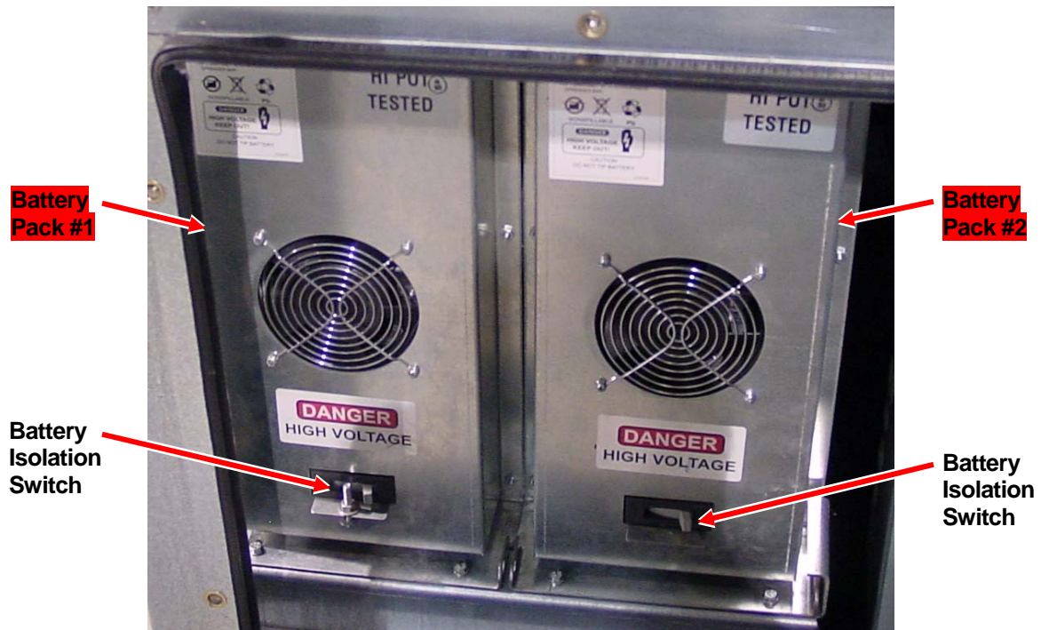
Figure 6. Battery Isolation Switch View, Lower Front of MT with Panel Removed
