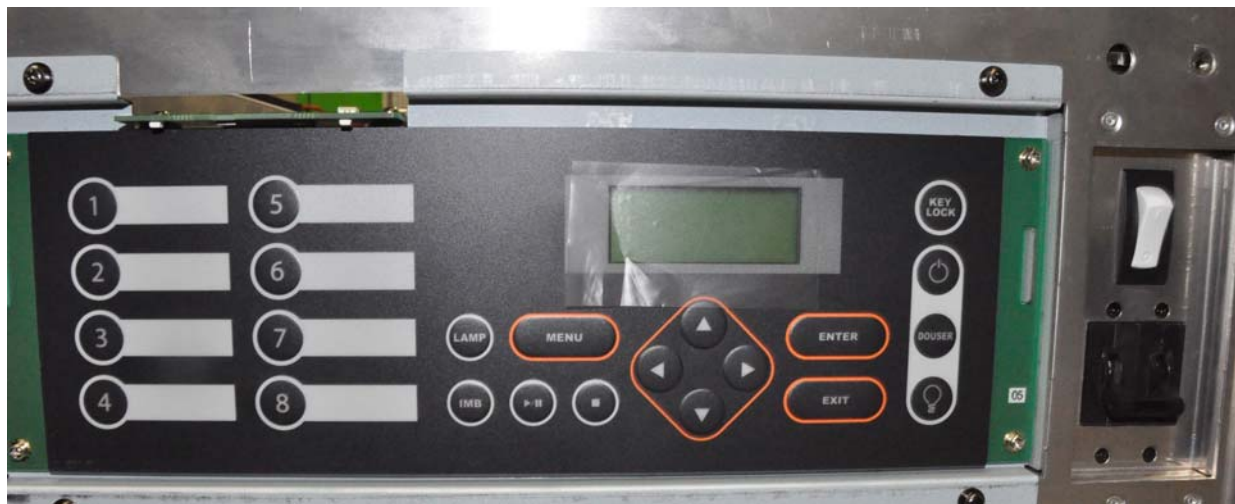
Figure 44: NEC 2000C Control Panel
