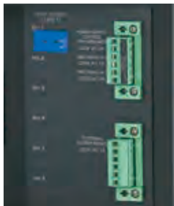
The external alarm terminal is optional.
