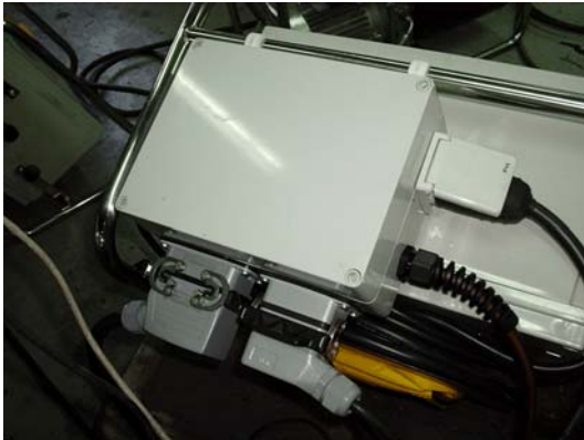
Figure 14a: Switch Box
