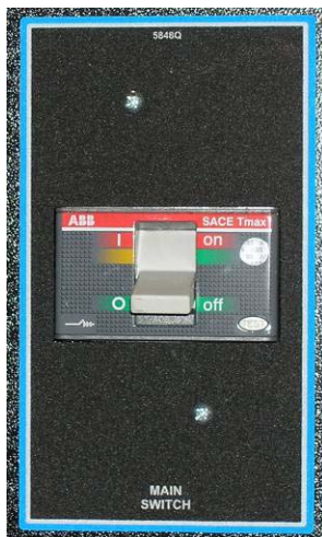
MAIN CIRCUIT BREAKER
