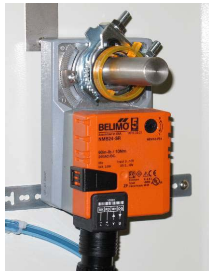
INTAKE DAMPER ACUTATOR
