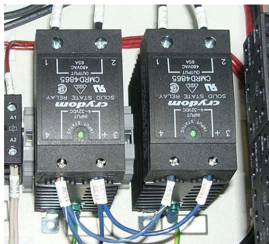
HEATER RELAYS SSR1 & SSR2
