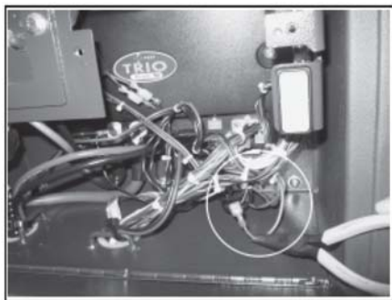
Figure 1 Jumper wire disconnected
