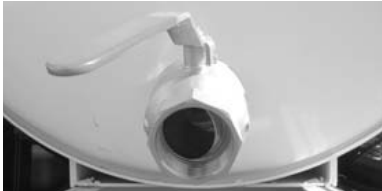
Figure 5-20. Check the drain valve before closing.
