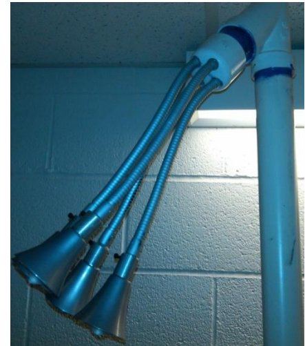
Figure 26 LED Flexible Fixtures
