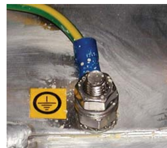
Place of connection of the earthing wire
