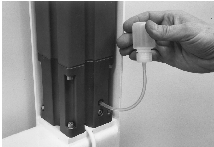
Figure 2.3 — Horizontal Damping Oil Installation
