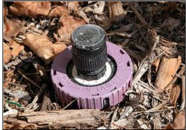
Recycled water sprinkler head with identifying cap
