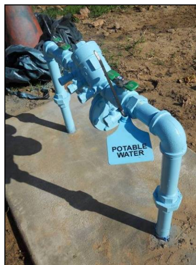
Potable water reduced-pressure backflow device with a POTABLE WATER identification tag
