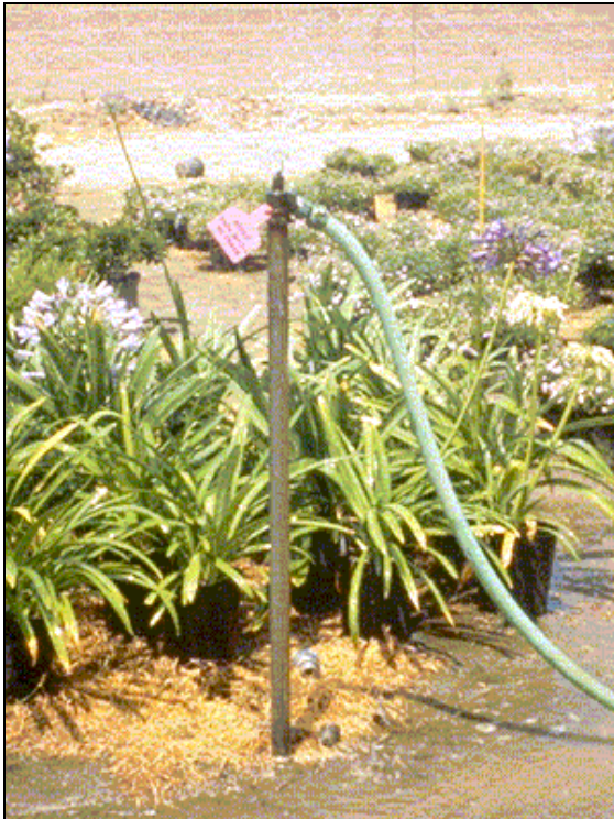
Hose bibs may only be used with recycled water in areas where they cannot be accessed by the general public (such as this commercial nursery), and even those must be properly labeled.
