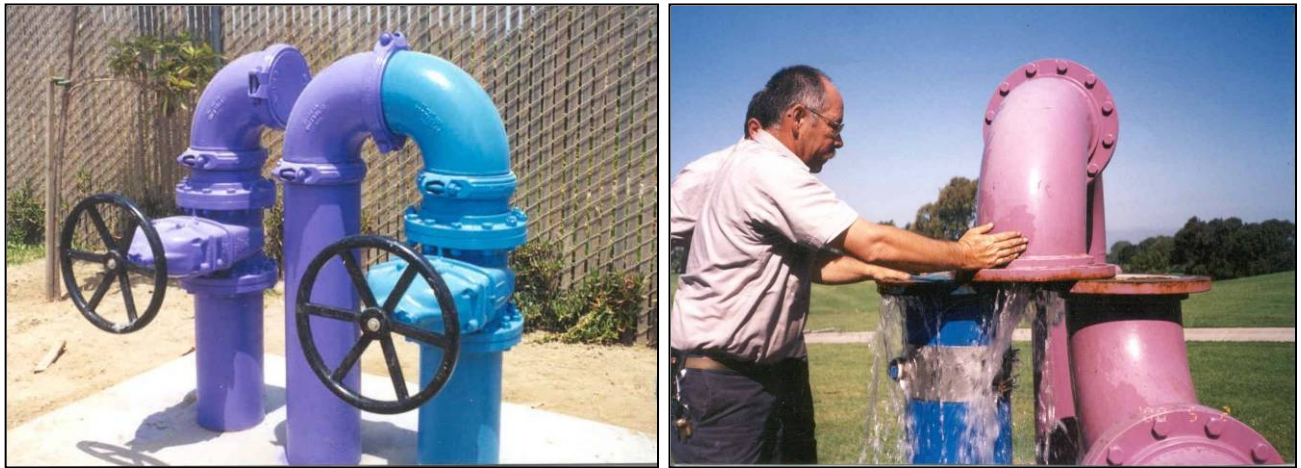
Example photos of existing "swivel-ell" assemblies for a back-up potable water supply.
