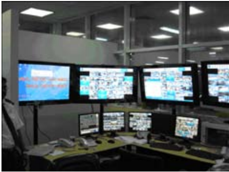
The central monitoring room is equipped with seven 42" flat screens and also seven 17" monitors..
