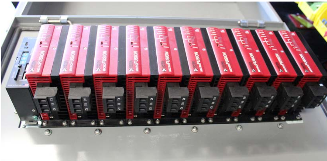
Figure 1: Controllers mounted through the side of the enclosure.
