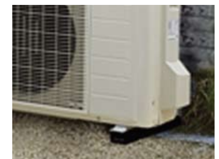
Piping connections for the outdoor unit are covered to make them less conspicuous.
