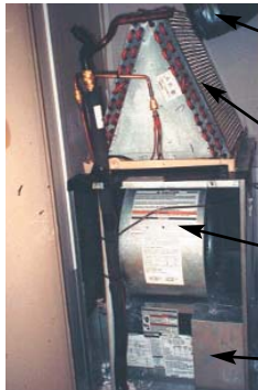
Inside a typical electric furnace closet
