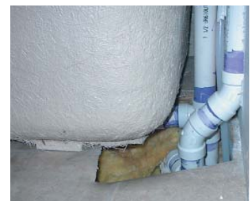
Hole in floor at plumbing penetration behind tub
