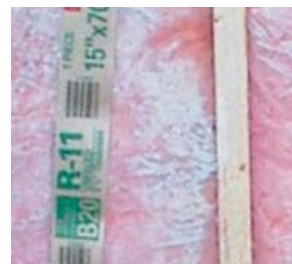
Fiberglass batt insulation
