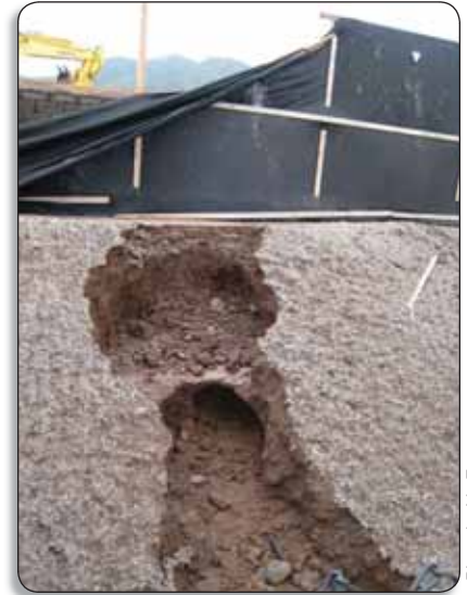
▲ Erosion at construction site
