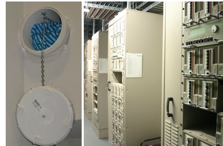
Left: One of the vast network of low technology 'mouse holes' that enable safe, simple and fire-rated connections between every space in the venue. The fire-rated bean bags in the tube (no it's not an old cleaning cloth) maintain the fire integrity of the wall.
