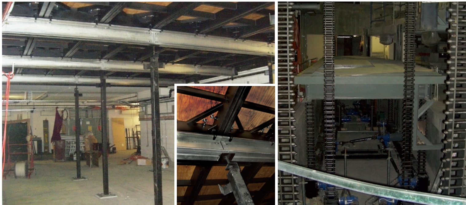
Left: The demountable stage system proposed by MTC's Craig Gamble and engineered by ShowTrek. Each removable deck module sits between two removable multi-sectioned joists supported by demountable pillars. The concept has been so well received by the industry that Jands and ShowTrek have already installed an identical system at the Queensland Performing Arts Centre. Inset: How all of the floor elements fit together. Right: The Serapid Linklift actuators that drive the three forestage lifts.
