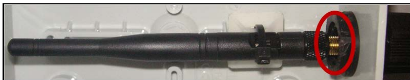
Figure 6-4 Outdoor installation; base of radio antenna showing inside the weatherproof box
