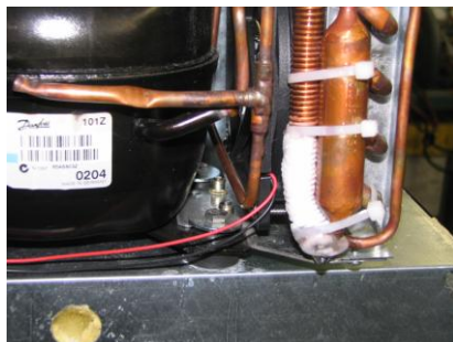
Ice accumulation around the cap tube usually indicates blockage.
