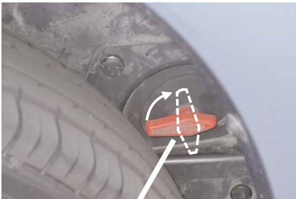
Manual Hydrogen Shut-Off Valve (Turn 1/4 turn clockwise to stop the flow of hydrogen.)
