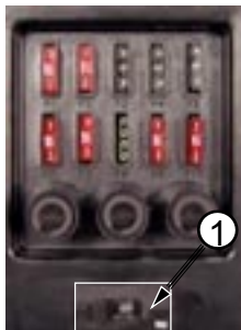
Figure 9 - Main Disconnect Switch
