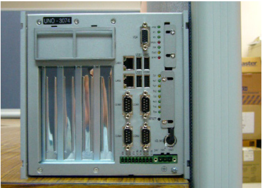
Figure 3.7: UNO-3074 Improper Installation (2)
