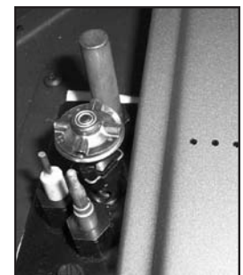
Figure 11. Ignitor assembly beside the burner.
