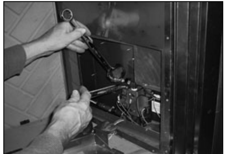
Figure 12.6 Turn off Gas Valve
