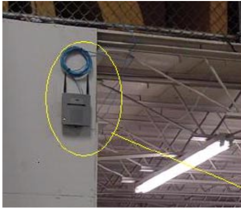
Figure 5-2 Access Point Installed on a Wall
