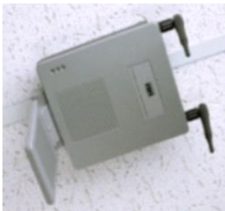
Figure 5-3 Access Point Installed on a Suspended Ceiling
