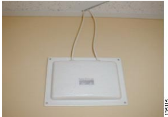
Figure 5-4 Patch Antenna Mounted on a Wall
