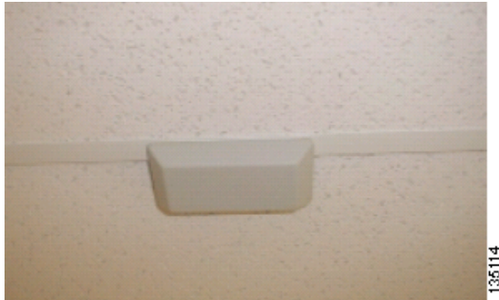
Figure 5-6 Patch Antenna Mounted on a Suspended Ceiling
