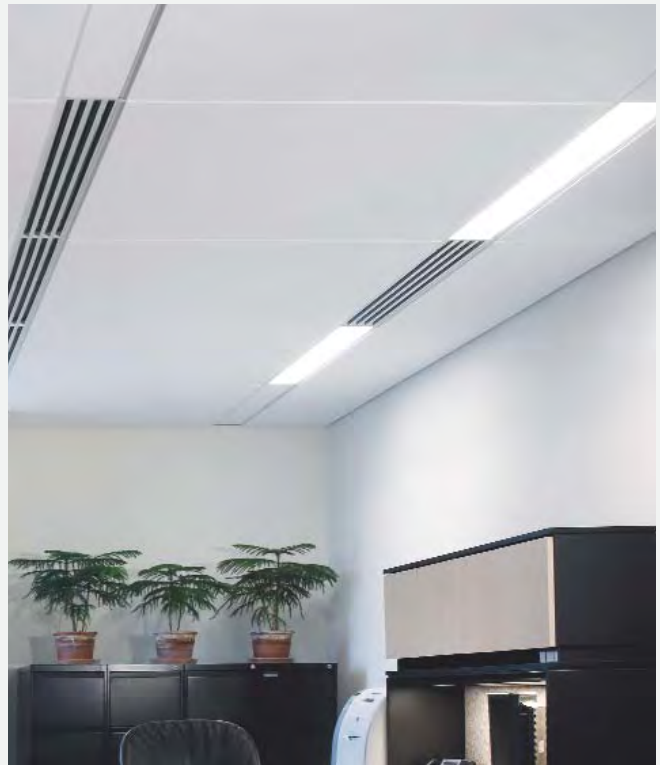
Optima 48" x 48" Tegular field panel and Optima Lay-In technical panels on Suprafine suspension system. Lithonia recessed light fixtures. Carnes air diffusers.
