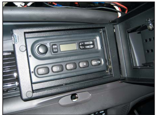
Connect AM/FM radio harness and antenna cable. Check radio operation. Snap radio into mount bracket.
