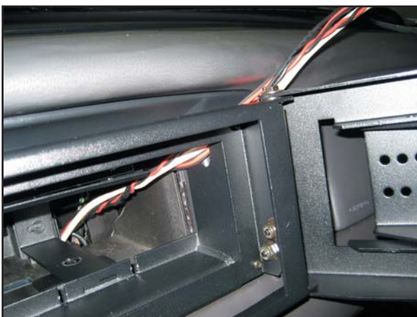
Run computer wiring through notch (top passenger side) and place monitor mount into dash cavity.
